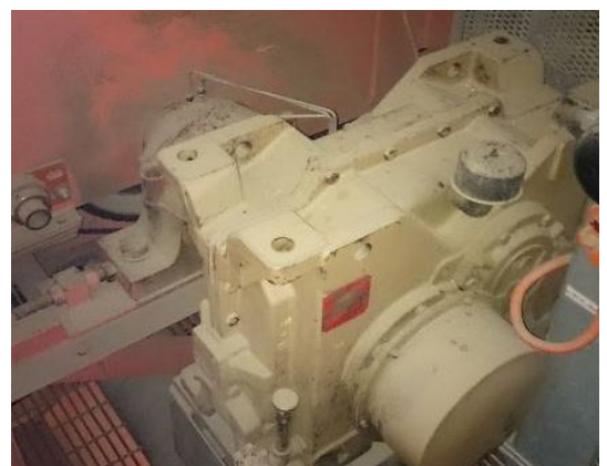
Bearing and seal grease lines
